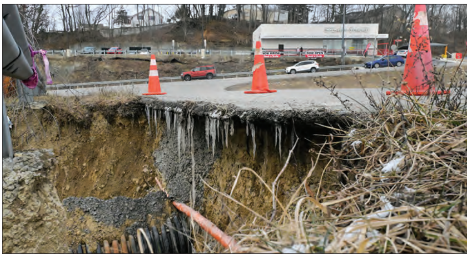
Ron Rittenhouse/The Dominion Post A DOH stormwater outlet has eroded the soil from beneath Star City's North Main Street, exposing a gas line.
